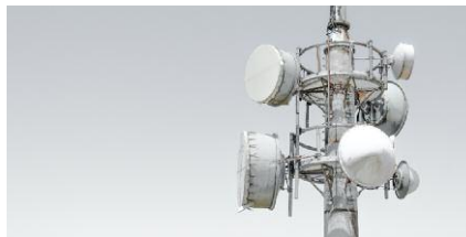
Microwave communications tower.
